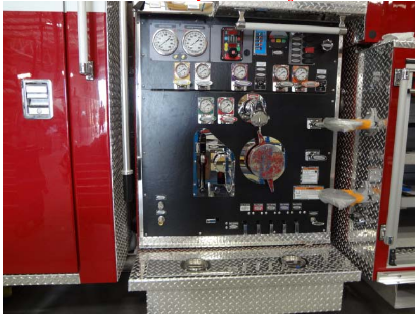
8/24/12 Driver Side Pump Panel/Running Board View
