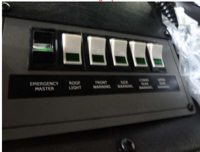
8/24/12 Cab Emergency Switches View
